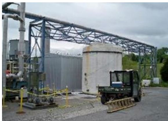
Figure 3.16. The Chromium Water Treatment System
